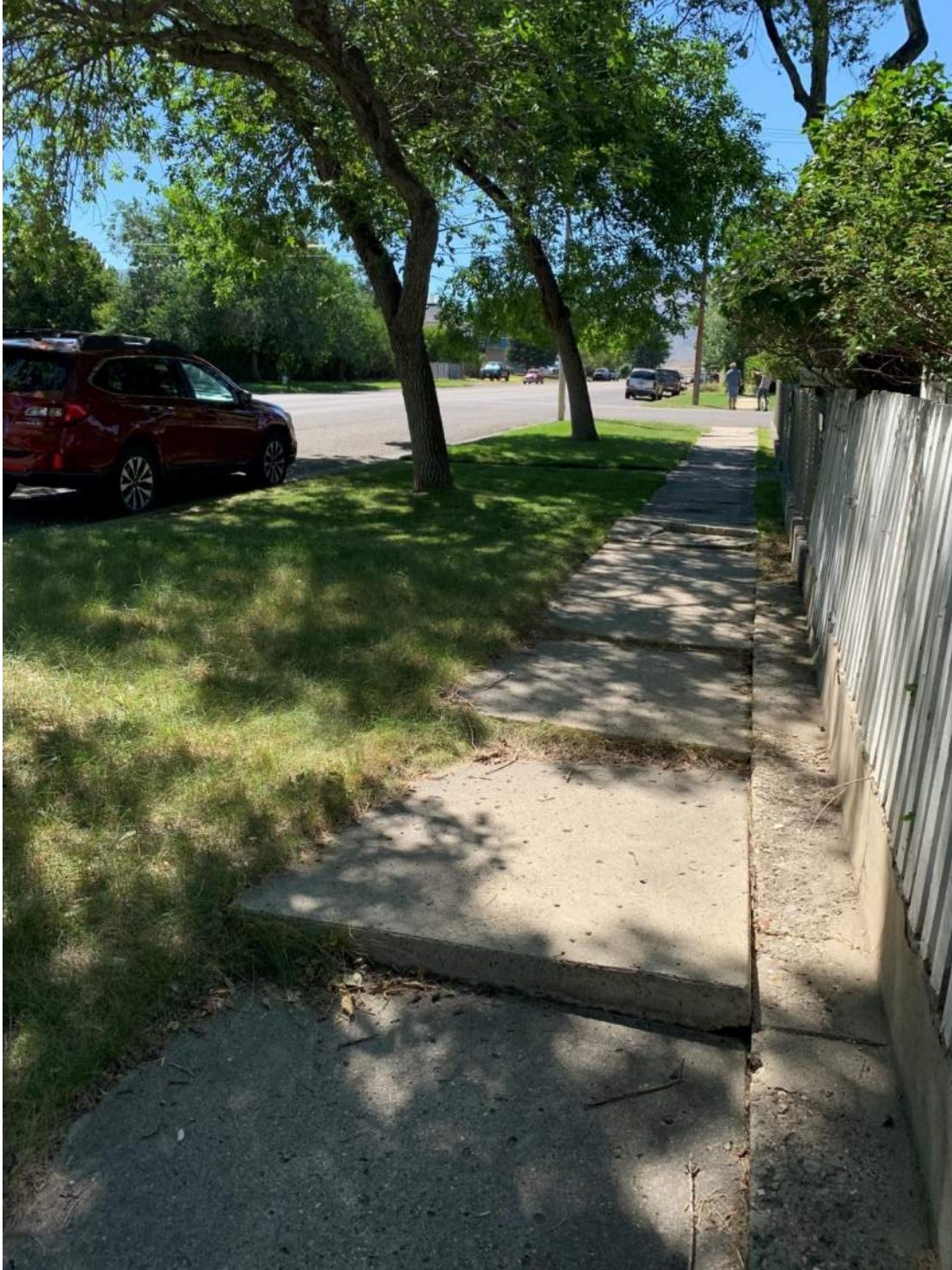
Figure 15. The trees and ample grassed parkway between the street and sidewalk create an attractive setting and comfortable place to walk; however, the sidewalk has shifted out of place creating a trip hazard for all users and inhibiting use by people with mobility disabilities. Concrete jacking and leveling services may be able to remedy this situation.
