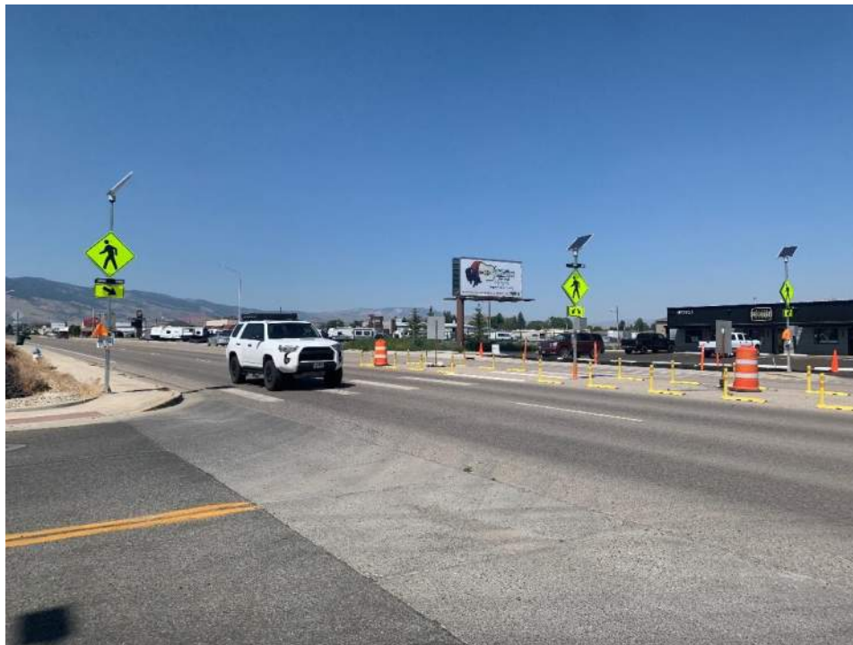
Figure 44. This temporary crossing of Big Horn Avenue will be replaced with a permanent crossing including crosswalk signage, pavement markings, pedestrian hybrid beacons, and a pedestrian refuge in 2024. Left turns will be prohibited on and off Big Horn Avenue at Freedom Street.
